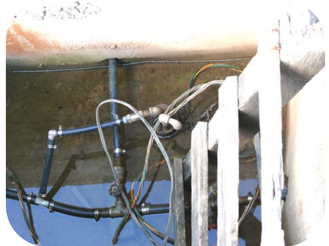
Photo 3. Wellhead in well pit
