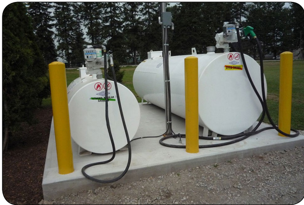
Figure 2. Proper storage of fuels reduces the risk to drinking water.
