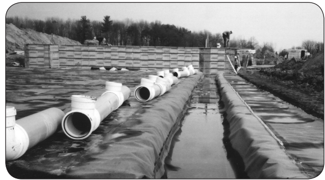
Figure 3. PVC pipe sections await connection and will eventually form a secure liquid manure transfer system from the in-barn tank to the external manure storage.
