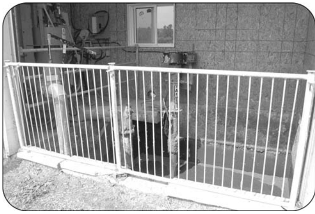
Figure 1. A liquid nutrient transfer system where liquid manure from the livestock facility is transferred to the anaerobic digester.
