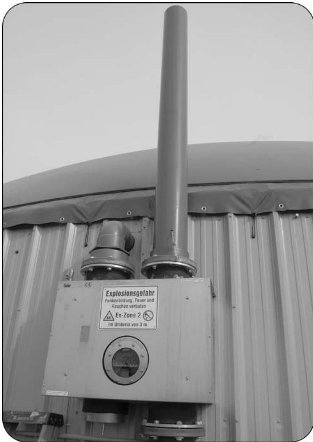
Figure 4. A freeze-proof over-under pressure relief valve installed on an anaerobic digester in Ontario.
