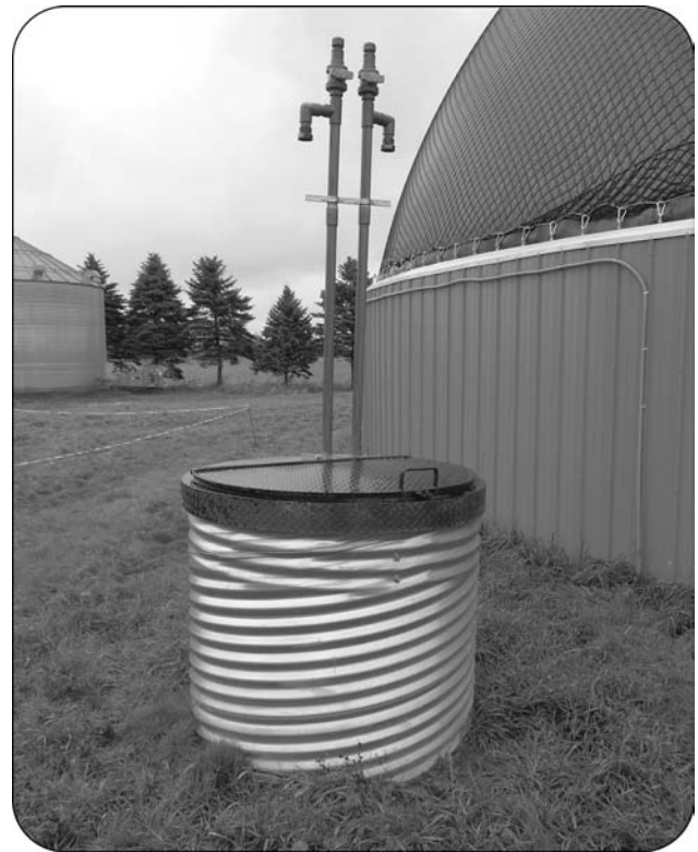
Figure 5. Access point to the condensation trap where the moisture removed from the biogas is collected.
