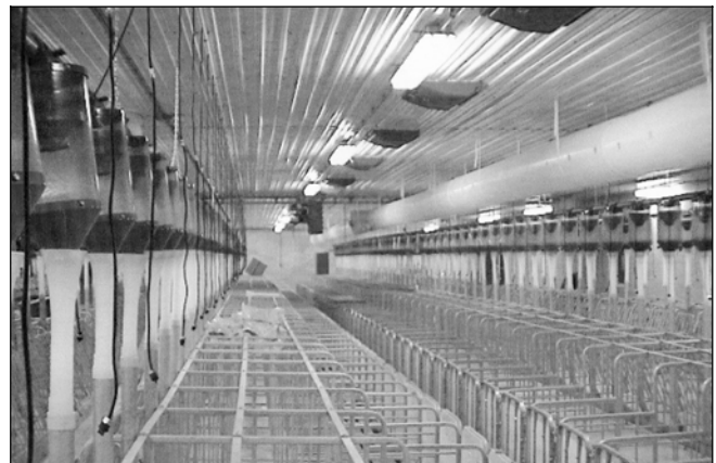
FIGURE 4. Vapour proof 4 ft. fluorescent fixtures in a swine gestation unit.
