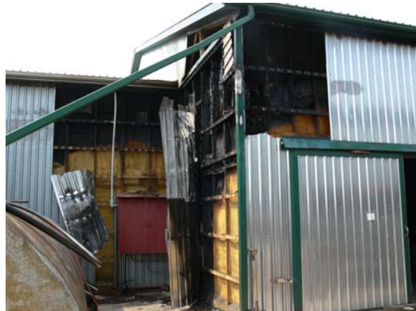
Figure 2: Parts of three walls were damaged in the fire. Note the blackened PUFI near the top of the wall because of a 'chimney-effect' inside the wall and horizontal spread of about 30 m (100') under eaves. The ignition point was in the centre of the picture near ground level.
